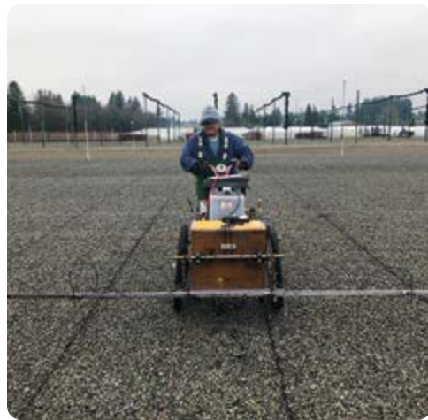
Augustin Moo paints perfectly straight lines to guide crews in setting off the newly potted trees
