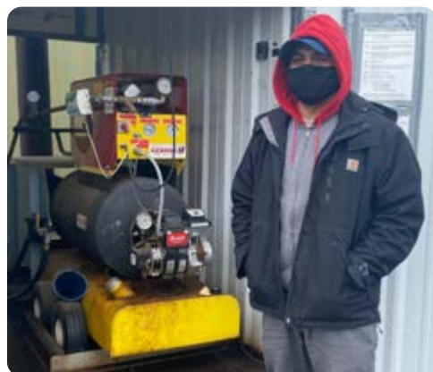
Hector Hernandez operates the steamer that sanitizes containers for reuse.
