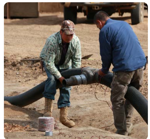
Rigoberto Elias and Austerberto Magaña work to install new drain lines in the sawdust.
