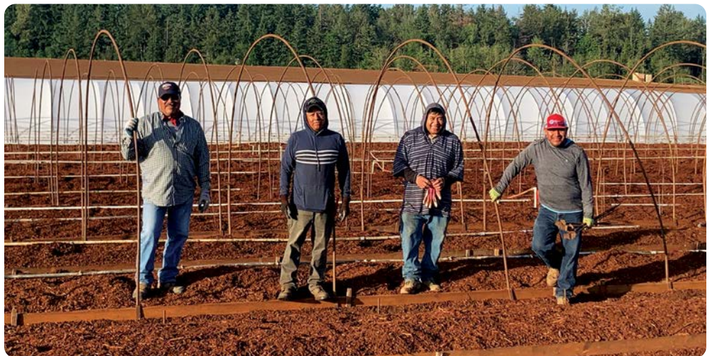
Agustin Galindo, Felipe de Jesus, Francisco Garcia, and Agustin Galindo-Acevedo have constructed polyhouses for years. They work at a fast pace to stay ahead of workers sticking cuttings in the newly completed houses behind them.
