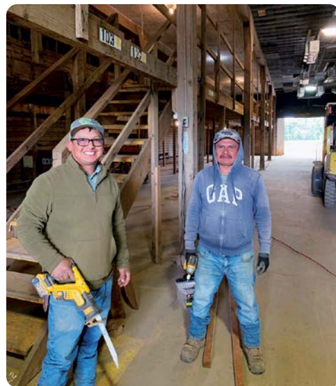
Rafael López and Martin González work on replacing bad boards in the cooler.
