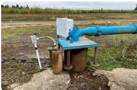
Example of a submersible pump well head. Pump and electric motor are both down the hole
