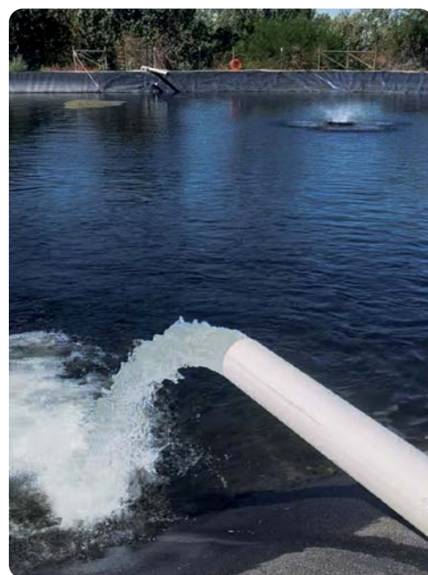
750 gallons per minute of fresh river water being pumped into the pond. The trees are going to love drinking this water!
